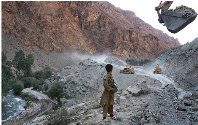
Workers are digging a road in Bamian Province to a site that is rich in iron ore, but that lacks the infrastructure to begin mining.
