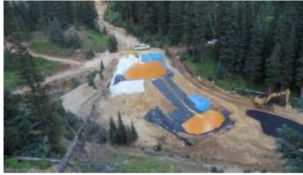
Yellow mine waste water from the Gold King Mine collects in holding pools in San Juan County, Colorado.
